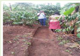
Fig. 13: Trenches to retain run off & improve water infiltration
